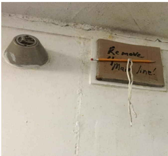
Photograph 4: Blocked Air Vent in a Cell
