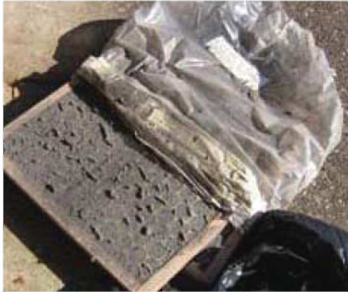
Image 3. Air filters from the general factory ventilation system, Building 5713
